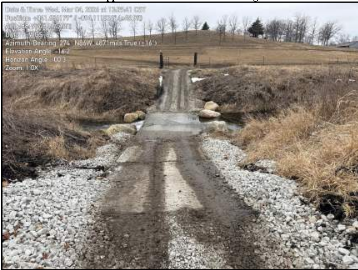
Vented ford crossing downstream of district to be lowered and reconstructed.
